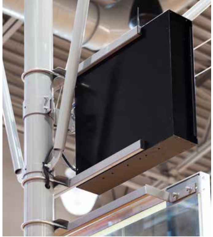
Location: Mendenhall Center Las Vegas, NV, Dealer: Hufcor Desert West, Mesa, AZ Photographer: Matt Oberer of mattophoto, Albuquerque, NM
